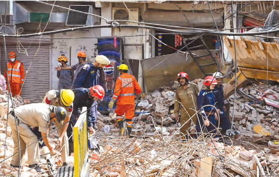
An excavator clears debris during search and rescue operations, a day after a five-storey building housing a boys' hostel collapsed, at Satya Niketan, in New Delhi PANKAJ KUMAR
