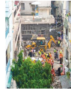
NDRF, Fire department officials at the site after a boys' hostel collapsed Delhi on Sunday
