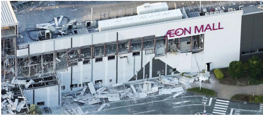
Damaged AEON Mall after an earthquake in Kashima, Japan
