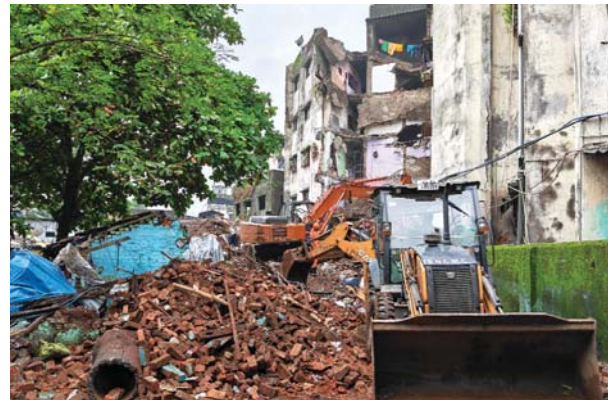
A portion of the Kohinoor Building in Balaji Nagar area of the powerloom town collapsed on late Thursday in Bhiwandi, Maharashtra on Friday. PTI
