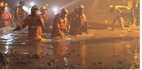
Rescue work in progress after a tunnel under construction at THDC India Limited's Vishnugad-Pipalkoti hydroelectric project in Chamoli district of Uttarakhand collapsed.
