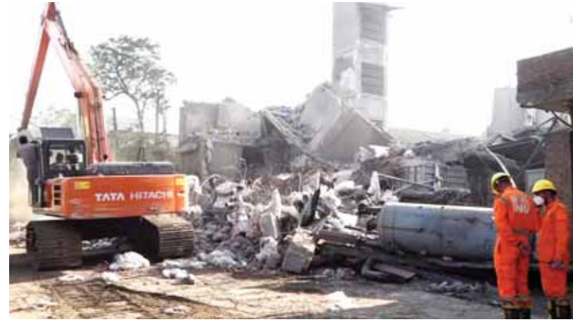
Rescue work underway after a multi-storey building of a textile factory collapsed in Ludhiana
