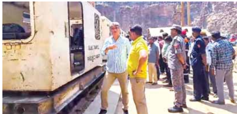
Rescue operation underway to trace workers trapped inside SLBC tunnel in Nagarkurnool
