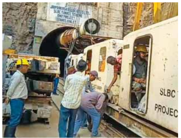
Emergency teams prepare for rescue operation to trace workers trapped inside Telangana's Srisaillam Left Bank Canal tunnel PTI
