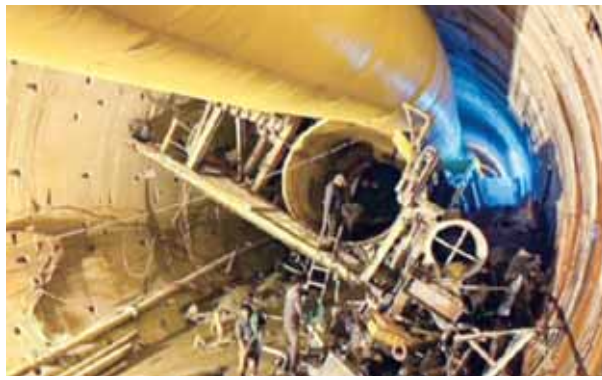
Rescue operation underway to trace workers trapped inside the partially collapsed Telangana's SLBC tunnel in Nagarkurnool, Telangana on Saturday
