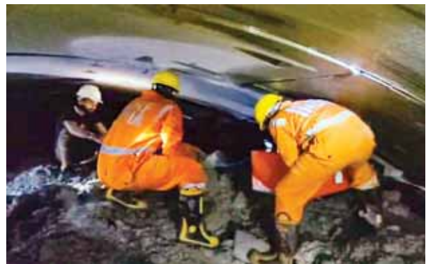
Rescue operation underway to trace workers trapped inside the collapsed tunnel in Nagarkurnool PTI
