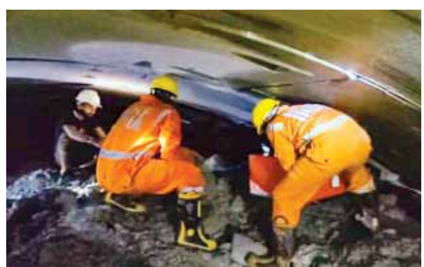
Rescue operation underway to trace workers trapped inside the collapsed tunnel in Nagarkurnool PTI
