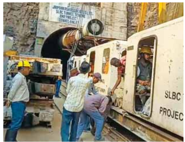
Emergency teams prepare for rescue operation to trace workers trapped inside Telangana's Srisailem Left Bank Canal tunnel PTI
