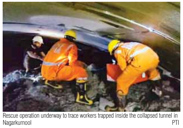
Rescue operation underway to trace workers trapped inside the collapsed tunnel in Nagarkurnool PTI
