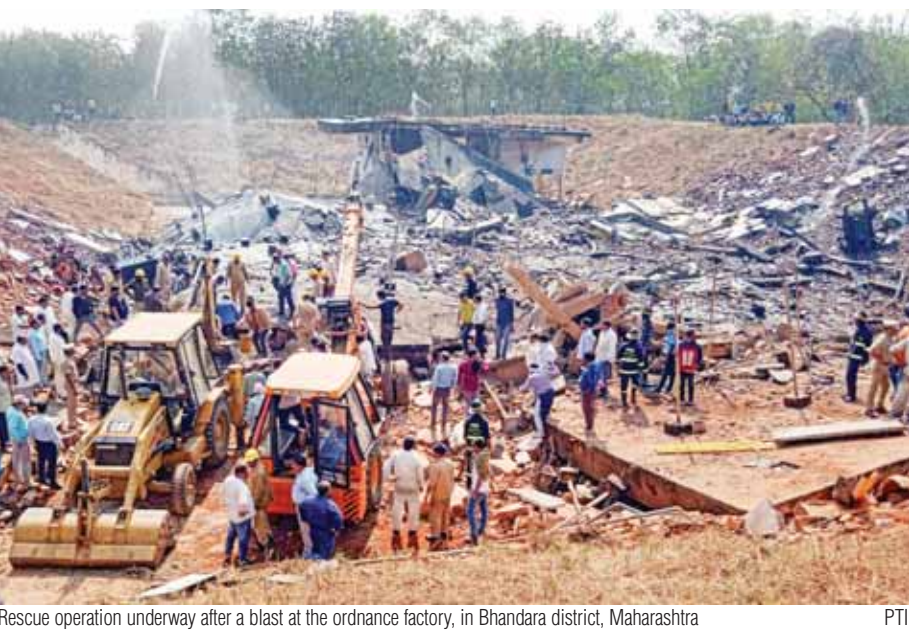
Rescue operation underway after a blast at the ordnance factory, in Bhandara district, Maharashtra
