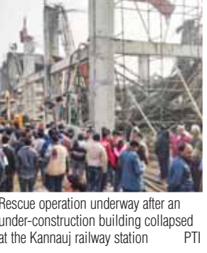
Rescue operation underway after an under-construction building collapsed at the Kannauj railway station
