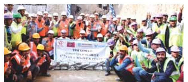
TBM achieves first tunnel breakthrough under the underground section of Corridor-2 of Kanpur Metro Rail Project.
