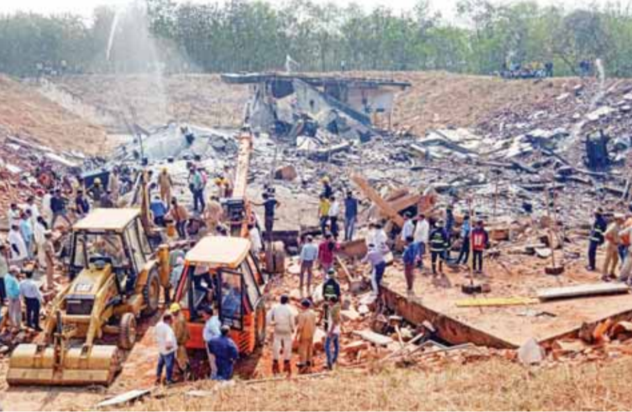
Rescue operation underway after a blast at the ordnance factory, in Bhandara district, Maharashtra
