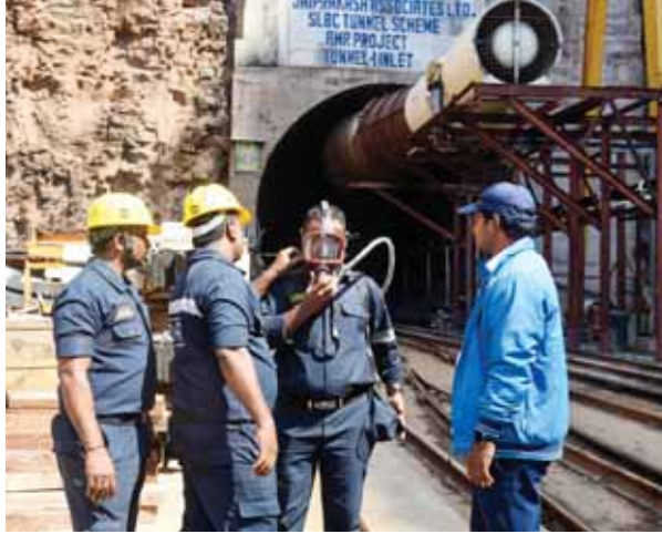
Rescue team at the Srisailem Left Bank Canal (SLBC) project site where a portion of the tunnel collapsed, in Nagarkurnool district. PTI
