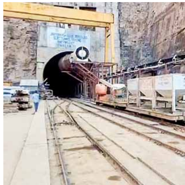
The project site where a portion of the tunnel collapsed in Nagarkurnool district on Wednesday PTI
