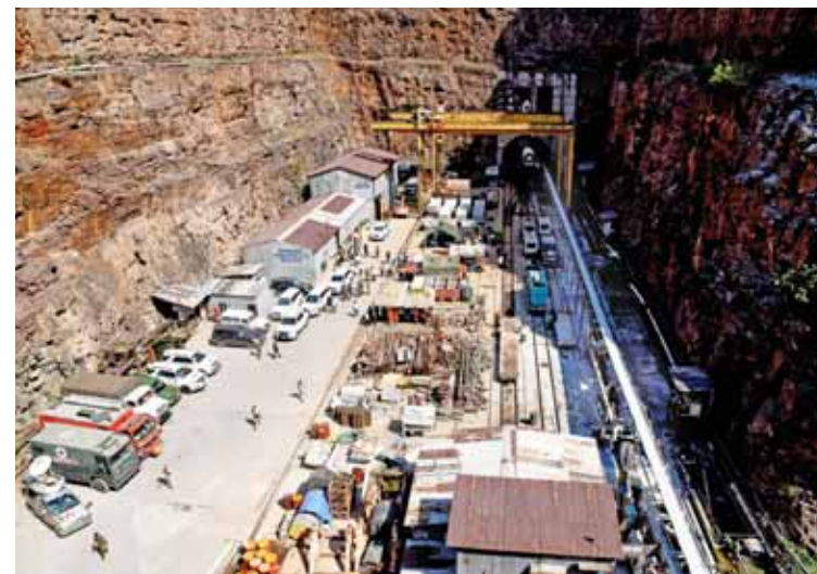
A rescue operation underway after a portion of the Srisailem Left Bank Canal (SLBC) tunnel collapsed in Nagarkurnool district
