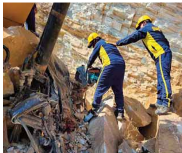
machine, resulting in the immediate death of the person inside. The SDRF had to cut through the JCB TO retrieve
