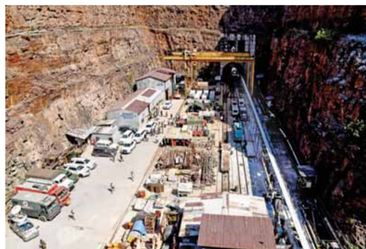
A rescue operation underway after a portion of the Srisaillam Left Bank Canal (SLBC) tunnel collapsed in Nagarkurnool district
