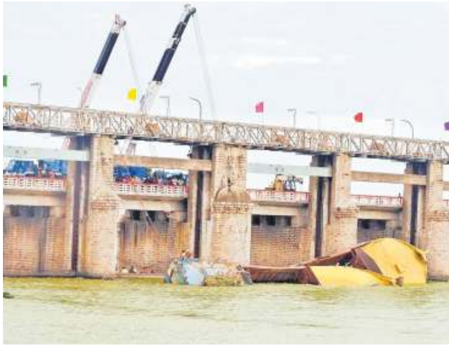
Workers removing the boats that are stuck at the gates of Prakasam Barrage in River Krishna in Vijayawada on Tuesday. The boats damaged crust gates and counterweights in recent floods (Photo: Ch. Vijaya Bhaskar)
