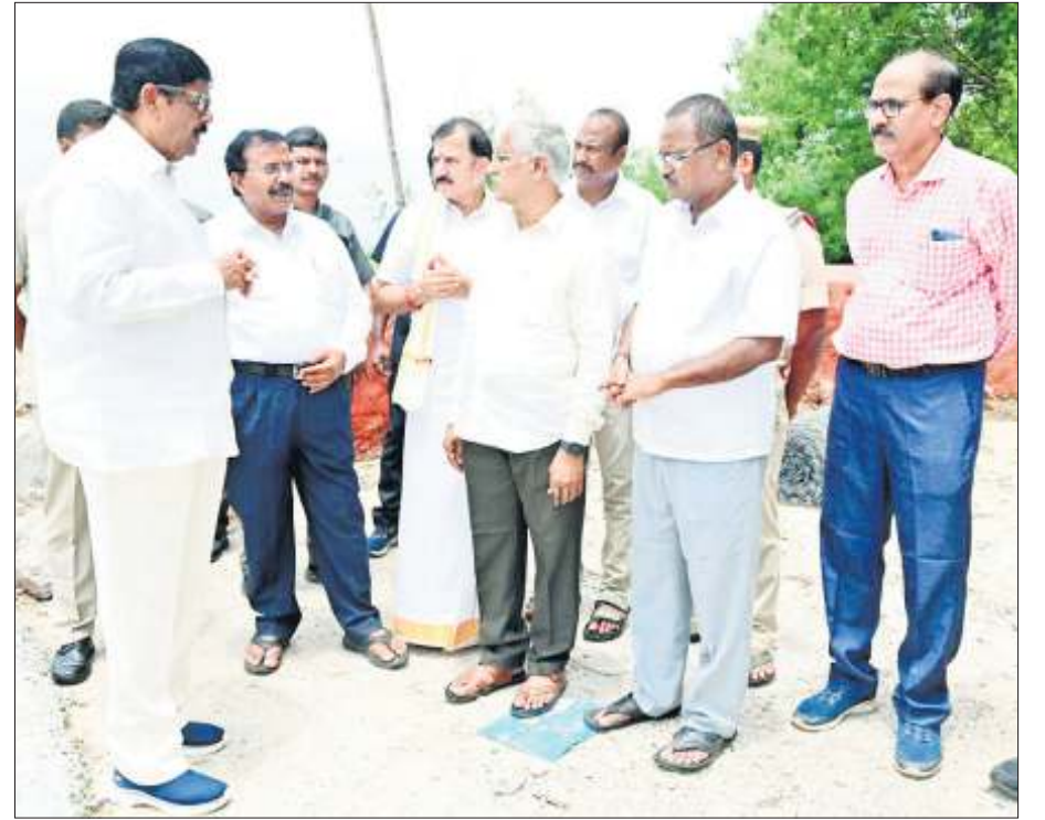
Endowments Minister Anam Ramanarayana Reddy, along with Principal Secretary S Satyanarayana, speaking to Durga Temple officials and engineers regarding the construction of the new retaining wall atop the Indrakeeladri hill on Tuesday
