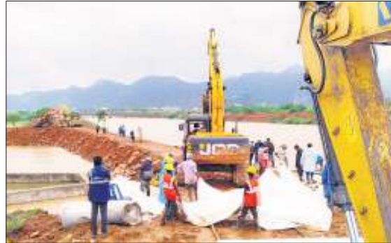
Megha Engineering experts at work to prevent floodwater leakage from the BDC at Shantinagar in Kondapalli of NTR district, on Monday.
