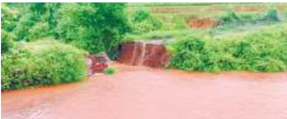
Collapsed bridge in Chapagedda village in Alluri Seetharamaraju district
