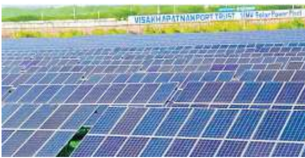
A view of the solar power plant at Visakhapatnam Port Authority
