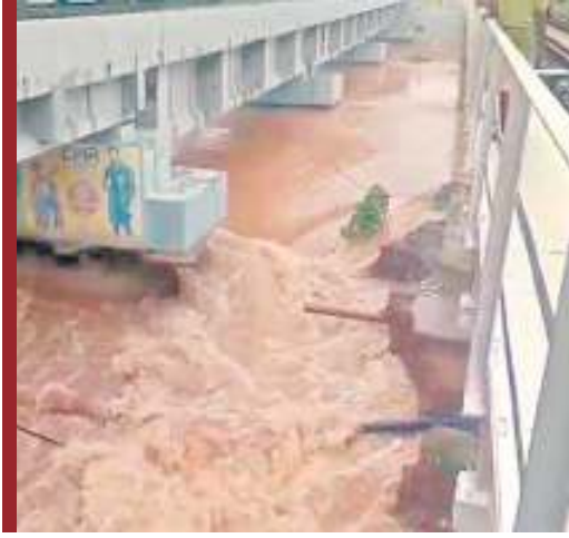
Over 36,000 cusecs of floodwater have entered the 'Budameru', but there is no proper channel for it to flow into the Enikepadu UT. As a result, the flood has submerged areas including Ajith Singh Nagar, Payakapuram, Rajiv Nagar, KV Kandrika, Prakash Nagar, Devi Nagar, and other localities within the Vijayawada Municipal Corporation limits, as well as Ambapuram, Jakkampudi, Rayanapadu, Kothuru Tadepalli, and other villages in the Vijayawada Rural Mandal.
