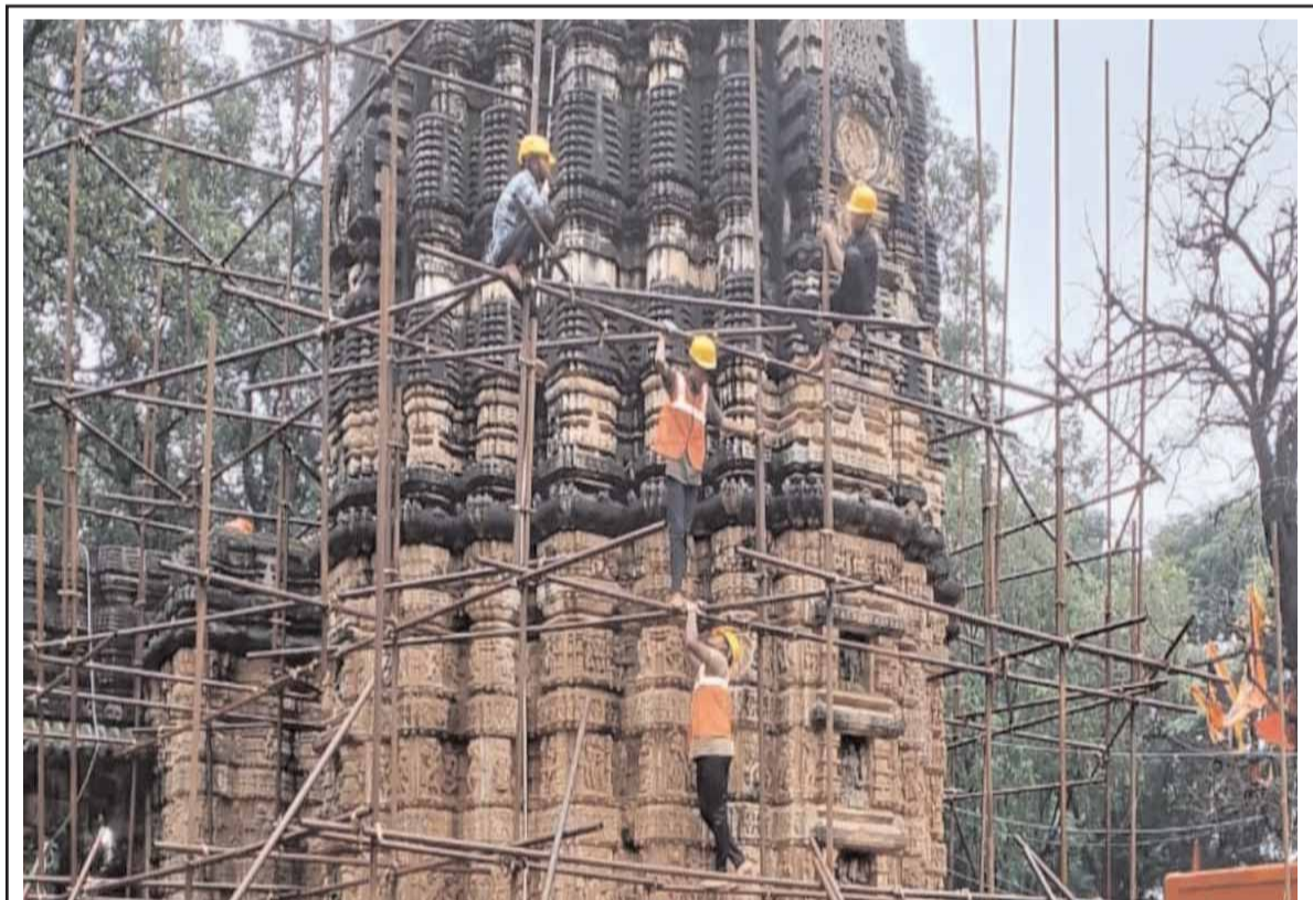
Restoration work of the Bhoramdeo temple in Chhattisgarh's Kawardha district is currently underway. The temple, a place of archeological importance, is being chemically treated. Also, water proofing work is being done.
