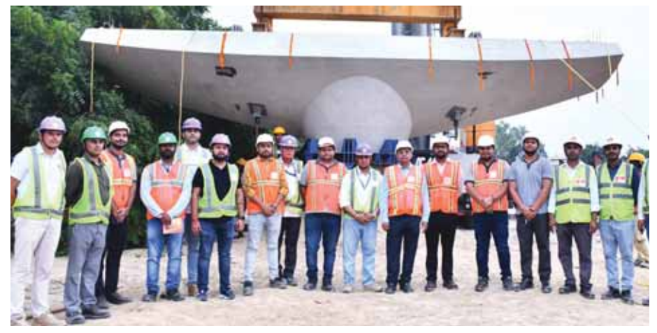
UPMRC started erection of pier caps for the elevated section of Corridor-2 on Monday.
