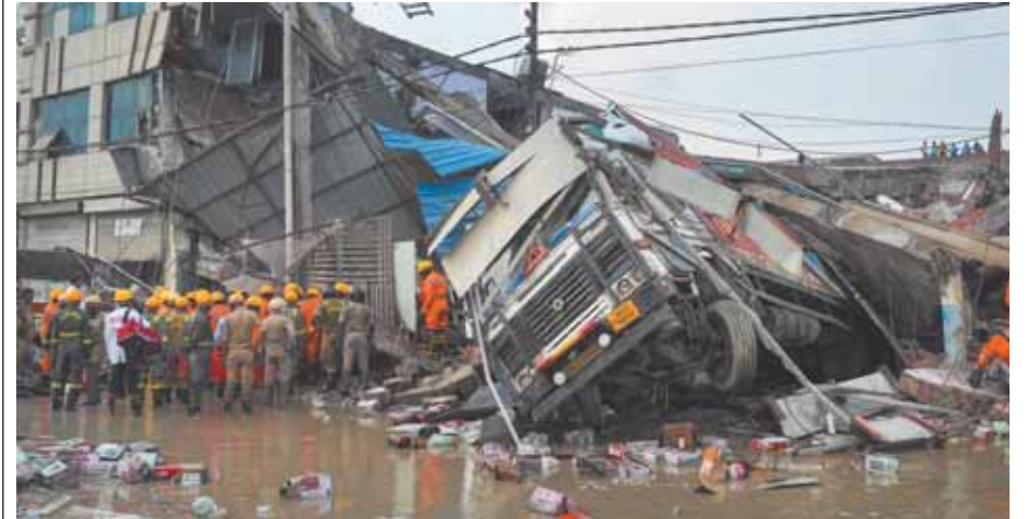
SDRF personnel conduct rescue operation after a building collapsed, crushing a truck under its debris, in Transport Nagar area of Lucknow on Saturday
