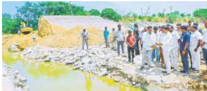
Revenue Minister Ponguleti Srinivas Reddy inspecting the repair works to Palair left canal under Kusumanchi mandal on Sunday
