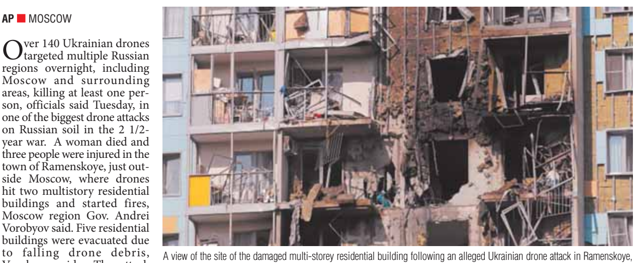
A view of the site of the damaged multi-story residential building following an alleged Ukrainian drone attack in Ramenskoye, outside Moscow region, Russia, on Tuesday.
