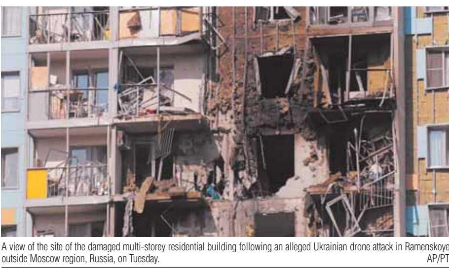
A view of the site of the damaged multi-story residential building following an alleged Ukrainian drone attack in Ramenskoye, outside Moscow region, Russia, on Tuesday.
