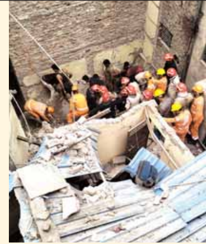
NDRF and Fire personnel conduct rescue operation as a house collapsed at Bapa Nagar (Karol Bagh) in New Delhi, on Wednesday
