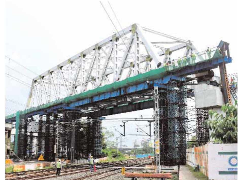
Officials and workers at their work after a girder was placed under the metro rail project at Habibganj in Bhopal on Tuesday.
