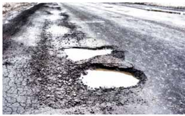
Chief Minister Atishi recently promised repair of all the damaged roads in the city by Diwali. The ministers of the Delhi government are currently visiting different areas of the city identifying damaged sections of the roads. Under the 'Pol-Khol' (expose) campaign of Delhi BJP, the party MPs, MLAs and senior leaders took to streets at 60 locations across the city, said a party statement. The party leaders and workers "exposed" the "media events" of
