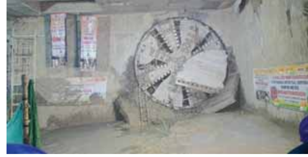
'Azad' TBM completes 330-metre section of the 'up-line' tunnel reaching Transport Nagar station.
