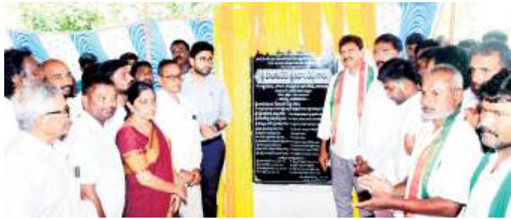
Revenue Minister Ponguleti Srinivasa Reddy laying the foundation stone for CC drains at SC Colony in Khammam on Wednesday
