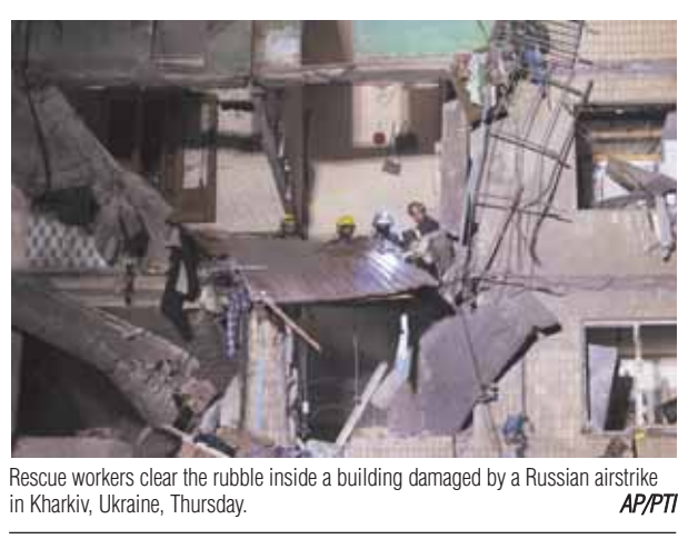
Rescue workers clear the rubble inside a building damaged by a Russian airstrike in Kharkiv, Ukraine, Thursday. AP/PTI
