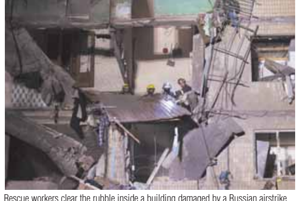
Rescue workers clear the rubble inside a building damaged by a Russian airstrike in Kharkiv, Ukraine, Thursday. AP/PTI
