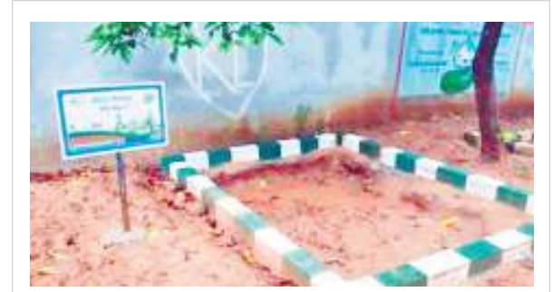
A rainwater harvesting pit arranged by the A.P. Federation of Resident Welfare Associations, at Simhapuri Layout in Visakhapatnam
