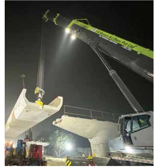
The erection of U-girders for the elevated section under the Kanpur Metro Rail Project began on Saturday.
