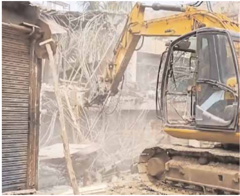
An excavator being used to demolish an illegal building at Kaiserbagh, in Lucknow, on Sunday
