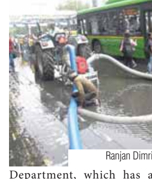
Department, which has a major chunk of roads under its jurisdiction, said they have repaired the permanent pumps and temporary pumps have been procured to drain out water. "The Delhi Traffic Police had identified 308 locations that had witnessed waterlogging last year. There are 214 locations under the PWD. Out of these, there were around 40 locations that required engineering intervention for
