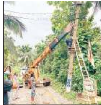
Power restoration works going on in APEPDCIL in the rain affected areas.
