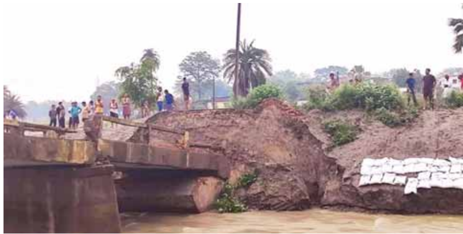
A view of the collapsed bridge amid heavy rain in Bihar's Siwan district on Wednesday
