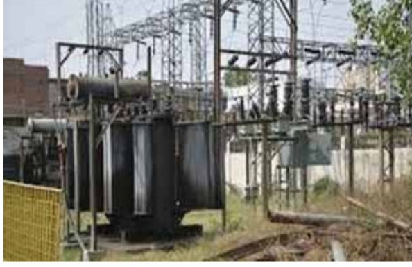
will be a radical improvement in the power supply system in the district. He said that at present the power supply is through a 132 kV line from the sub-station located in Bilaspur. Due to the long distance, technical problems have been disrupting the supply besides low voltage issues. The sub-station will also facilitate smooth power supply to the neighbouring state of Jharkhand. Besides, 176 new additional transformers have been installed in the district to improve the power system. Bhagat said the district has received approval for additional 274 transformers to improve the power system in the district. Of these, 176 have been installed.
