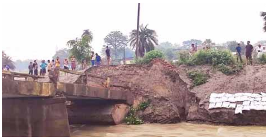
A view of the collapsed bridge amid heavy rain in Bihar's Siwan district on Wednesday
