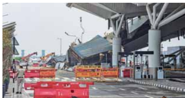
Restoration and relief work underway at the Terminal-1 of the IGI Airport where a canopy collapsed amid heavy rain in New Delhi
