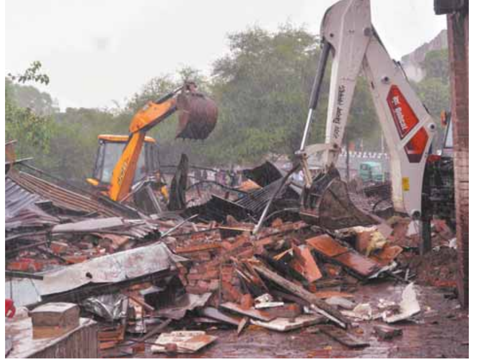
Bulldozers in action on Thursday to demolish the 'phool mandi' which had come up unauthorisedly on Hussainabad Trust land in Kanchan market area of Chowk
