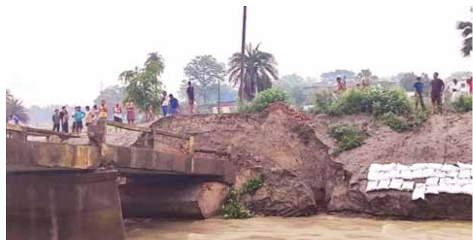
A view of the collapsed bridges amid heavy rain in Bihar's Siwan district on Wednesday
